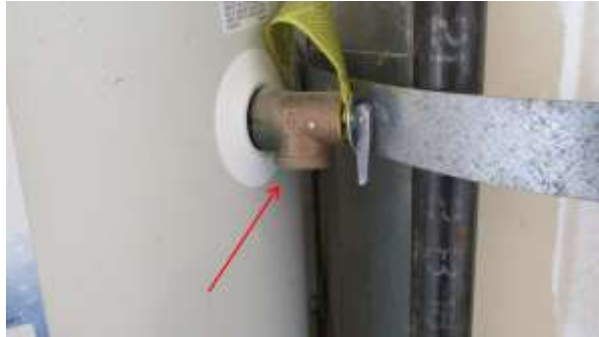
TPRV is missing discharge pipe.
