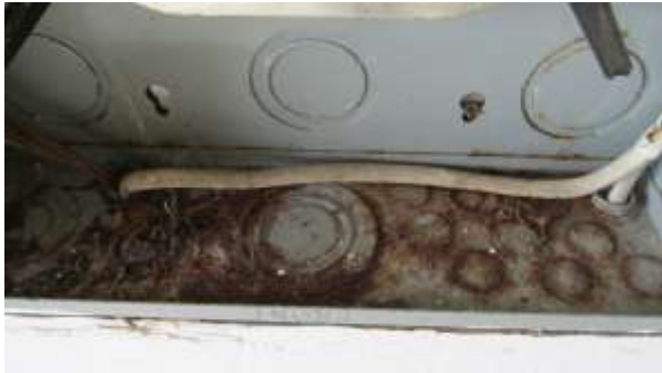
Corrosion in Main Electrical Service Panel
