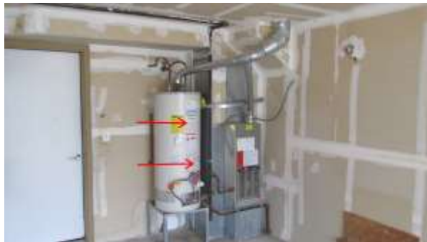
No earthquake straps around the water heater.
